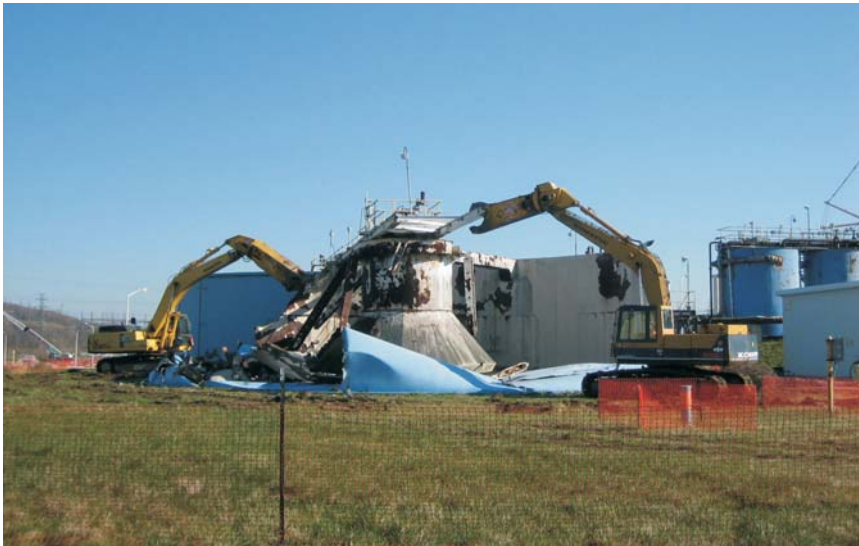
Shutdown of the gaseous diffusion uranium enrichment process and demolition of structures no longer needed such as the X-616 Liquid Effluent Control Facility
