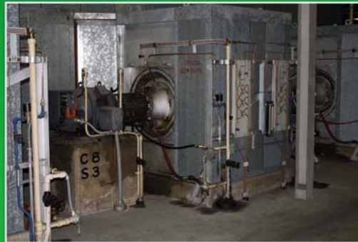
Compressors are housed within a heated enclosure for temperature control.
