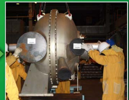
Compressor is lowered to the Operating floor to await shipment to the Nevada National Security Site (NNSS) for disposal.
