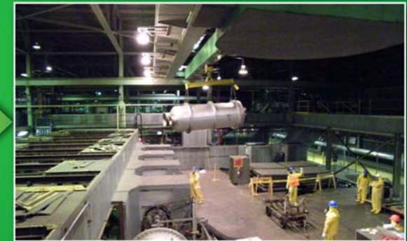
Once removed from the cell housing, the converter is moved to an open area.
