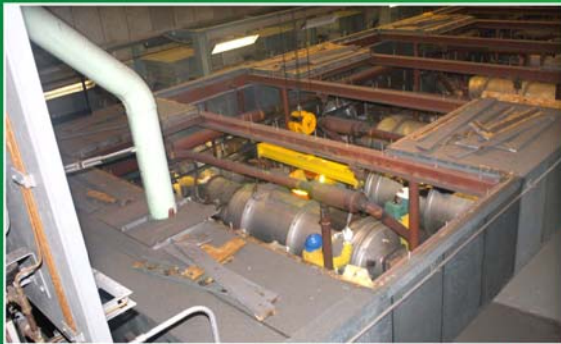
The overhead bridge crane and a converter lifting fixture is lowered into place and attached to the converter.
