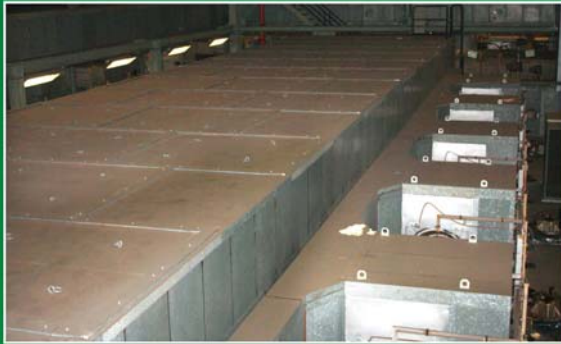
Cell components are housed within a heated enclosure for temperature control.
