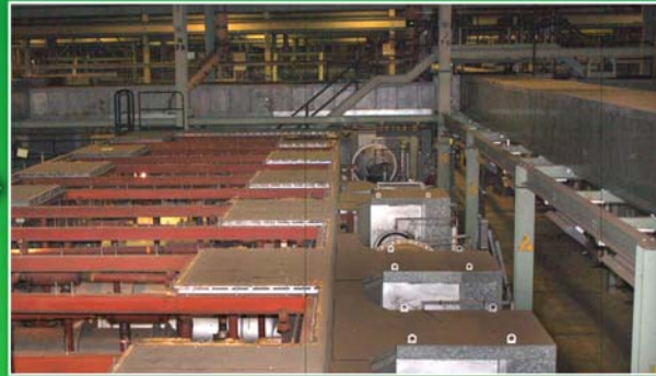
Hatch covers removed to allow access to the converters.
