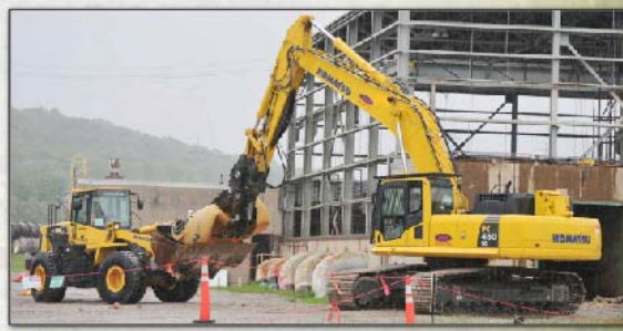
2011 A holding tank is removed from the Pump House in X-630 Recirculating Cooling Water Complex. This was the first building taken down by Fluor-B&W Portsmouth LLC under the $2.1 billion Decontamination and Decommissioning contract awarded by the Department of Energy in August 2010.
