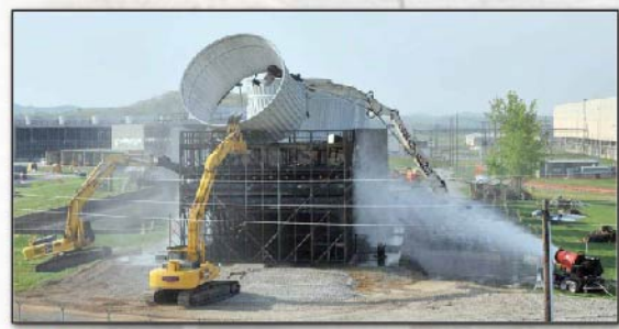
2010 Demolition begins on the first of four cooling towers (tower C) in the X-633 Recirculating Cooling Water Tower Complex. Each tower was 360 feet long, 72 feet wide and 45 feet high and resulted in the disposition of more than 738,000 cubic feet of waste.
