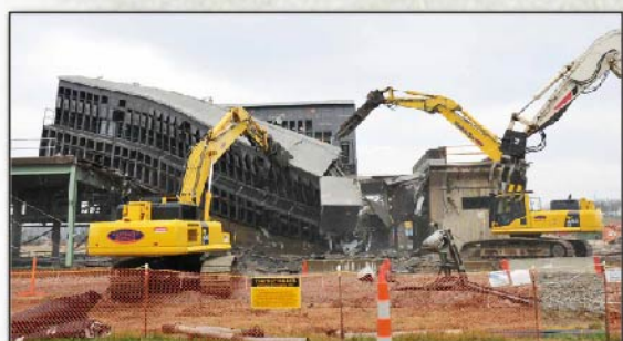
2010 The East Switch House was one of several large components removed from the 20-acre X-533 Switchyard.
