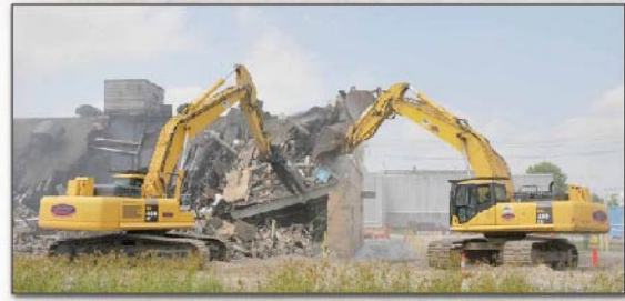
2010 Shears cut through the southeast corner of the X-760 Chemical Engineering Building.
