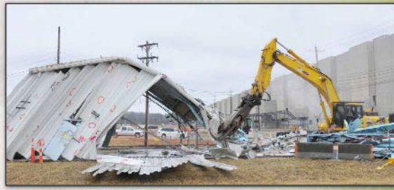
2011 With the last structural supports weakened, the X-334 Transformer Cleaning and Storage Building is brought down.
